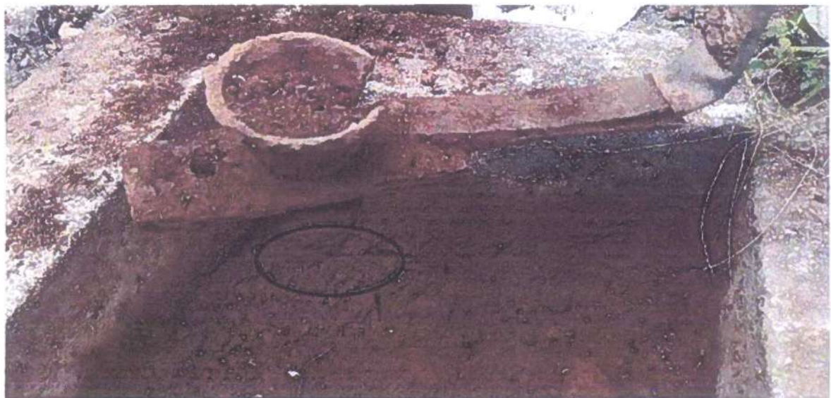
Neutral earth strip from transformer is detached from earth conductor, therefore transformer neutral earth was floating posing a great danger to the mains supply users
